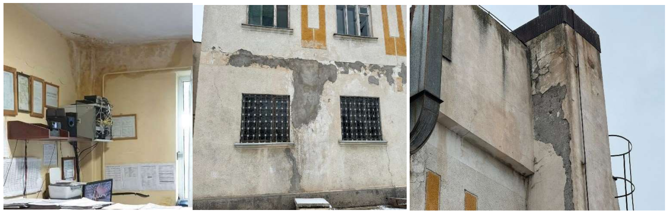
Figure 6 Visible deterioration of the existing ZFD's buildings
